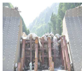
Fig.2 Steel open dam was partially collapsed by large rocks
