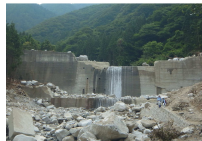
Figure 2: Collapse of concrete sabo dam
