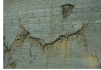
Figure 3: Cracks on the rear face of the dam
