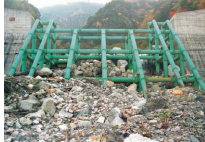
Photo 11: Status immediately after capturing debris flow
