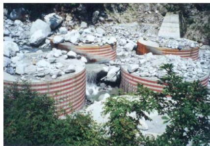
Photo 13: Status immediately after capturing debris flow
